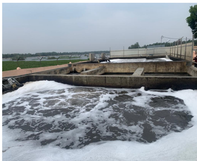
Fig. 4: MBBR aeration zone
